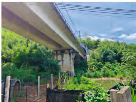
K753+820 混凝土开裂、破损边坡防护
